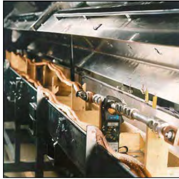
Test of terminals.
