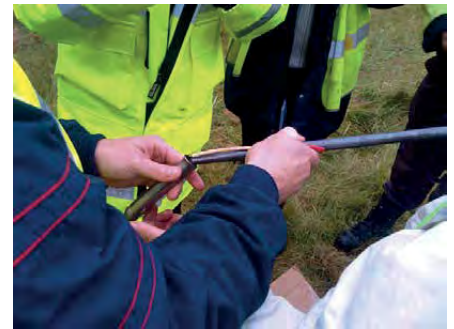
3. The earth line is locked to the hardened steel tip with the leading rod.
